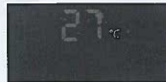
Standby with no Key lock
